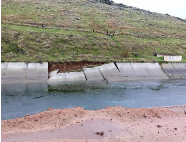
Friant-Kern Canal subsidence
