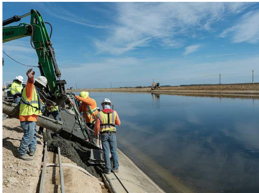
Workers repair a section of the California Aqueduct in Kern County. (Source: DWR)
