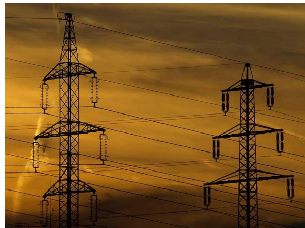
Electric lines (Photo by Petr Kovar from FreelImages )
