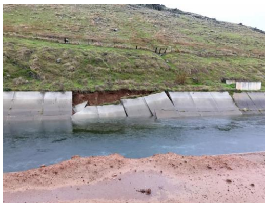
Ground subsidence along the Friant-Kern Canal.
